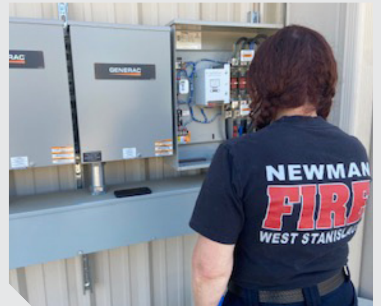
Newman Fire Department’s grant funded the installation of transfer switches at their town’s fire house to help when power goes out.
