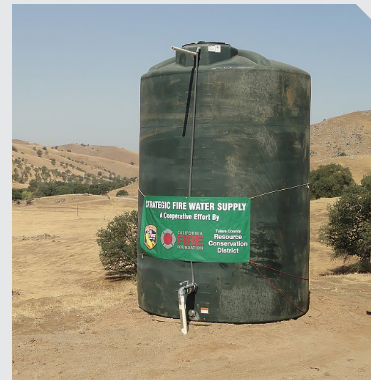
Tulare County Resource Conservation District & Sequoia Fire Safe Council’s funding helped purchase and site 5,000 gal. water tanks in strategic fire prone areas for rapid water deployment and suppression support. Over 4,500 residents populate the “at-risk communities” within the grantee’s service area, with eight communities within wildlands being designated as under-resourced.
